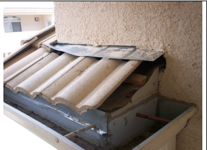
Damaged roof flashing and missing shingle
