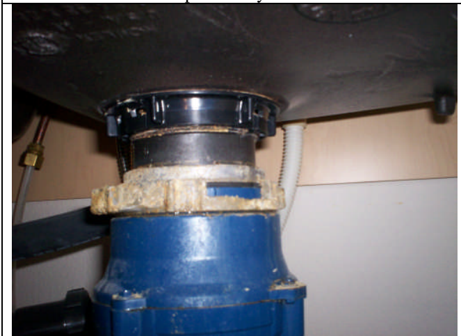
Water leak at connection to disposal
